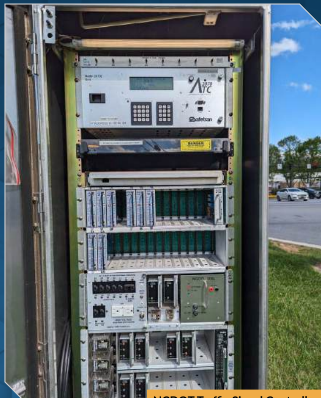
NCDOT Traffic Signal Controller
