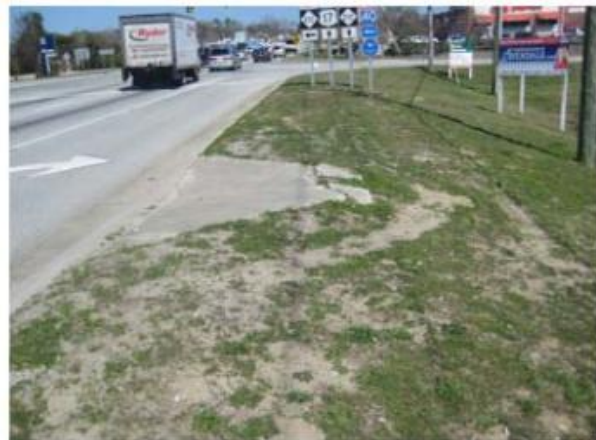
Figure 16: Broken Wheelchair Ramp along E side of US 17
